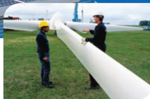
RIGHT: Construction of wind powered electricity generators at Crookwell, NSW. Photo by: Gregory Heath
