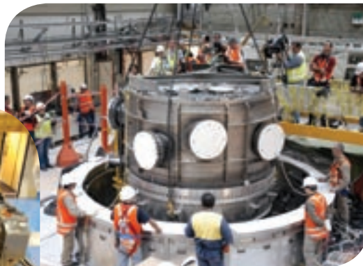
Construction of OPAL-The reflector vessel is lowered into the reactor pool, under the watchful eye of the media. Photo by: ANSTO www.ansto.gov.au
