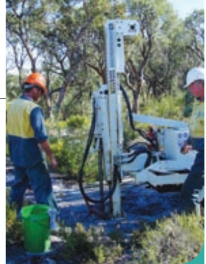
Drilling a bore hole to measure soil water distribution and groundwater levels on the Gngangara aquifer.
