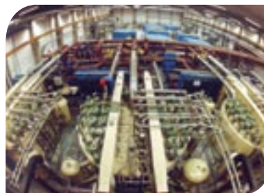
The central refrigeration plant supplying HERA's proton ring with liquid helium. (Source: DESY in Hamburg). Photo by: DESY in Hamburg, Helmholtz association, DESY - Deutsches Elektronen-Synchrotron.
